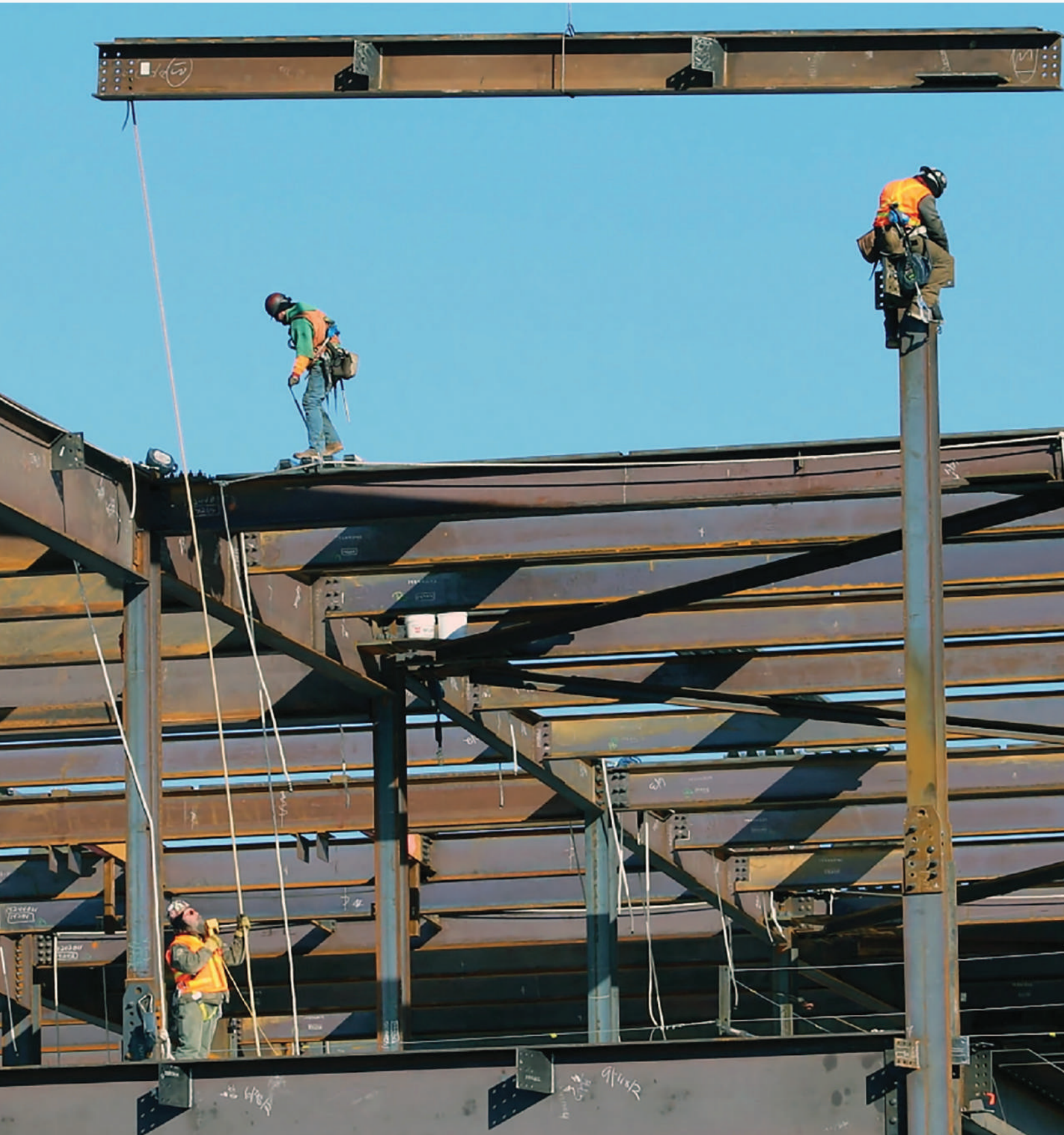
Construction workers at John F. Kennedy International Airport guide a steel beam into place.
