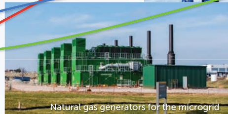
Natural gas generators for the microgrid
